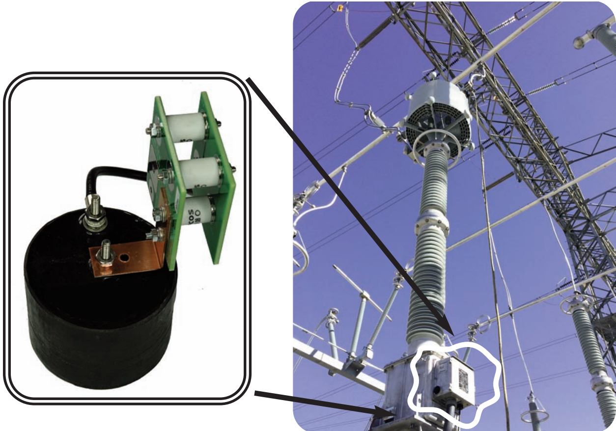
Close Up of Smart Gap Mounted on the Drain Coil (Left) and Location Inside Coupling Capacitor / CCVT Base Housing (Right).
