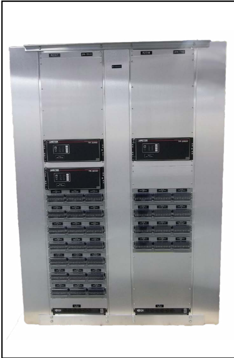
Double Lucasey Rack with TR-3000 Digital Fault Recorder and ABB FT-19R test switches.
