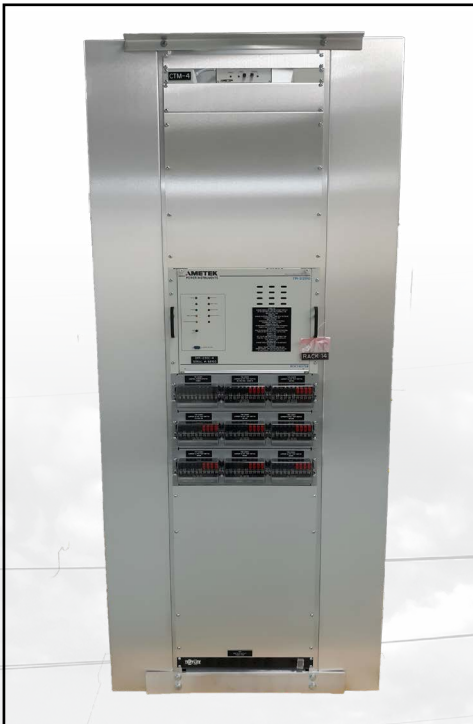
Single Lucasey Rack with TR-2200 and ABB FT-19R test switches.
