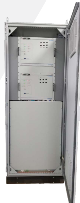
Rittal Cabinet with TR-2200.
