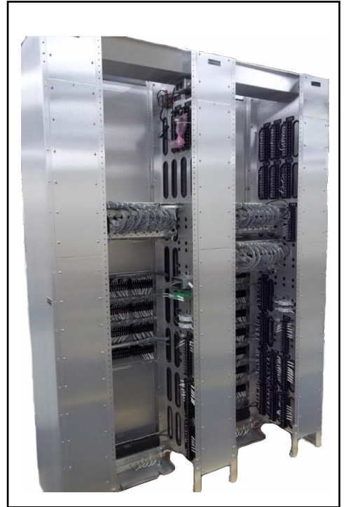
Rear view of Lucasey Rack with TR-3000, ABB FT-19R test switches and GE EB-25 terminal blocks.
